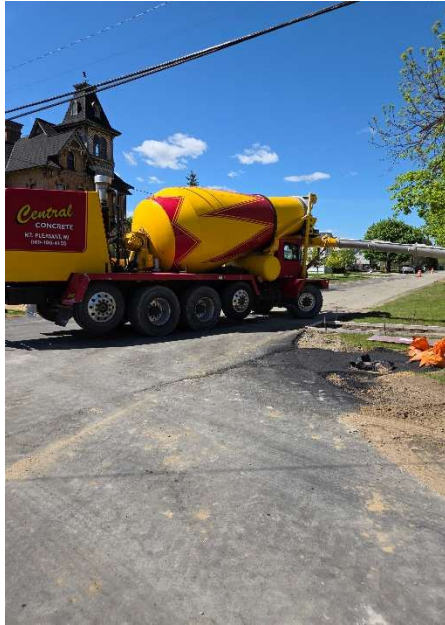
Photo 1: Phase #1 – Concrete sidewalk and driveways placed on N. Delaware, Tamarack and Berea
