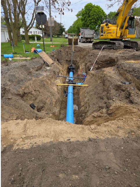
Photo 1: Phase #2 – Water Main placed on Prospect St. to the east end of the street.
